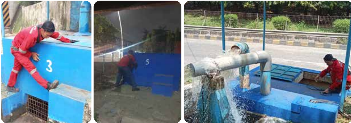
Lokasi pekerjaan Perawatan Pompa pengendali banjir di Cawang Interchange , Tanjung Priok, dan Gerbang Tol Pluit. The Maintenance of Flood Control Pumps were carried out at Cawang Interchange, Tanjung Priok, and Pluit Toll Gate.
