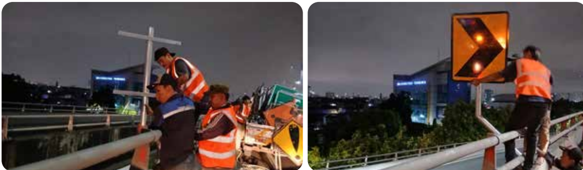
Lokasi pekerjaan Perawatan Sarana & Prasarana Jalan Tol dilaksanakan pada lokasi KM 5.000 ruas North-South-Link dan KM 18.700 ruas Harbour Road . The maintenance of Toll Road Infrastructures & Signs were carried out at KM 5,000 of North-South-Link section & KM 18,700 of Harbour Road section.
