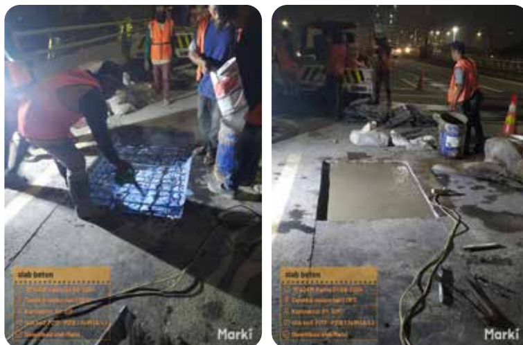
Lokasi perbaikan Grouting Plat Lantai Jembatan (beton Slab) di laksanakan spot by spot pada lokasi ruas North-South-Link . The Bridge Floor Plate Grouting (concrete slab) repair was carried out spot by spot at the North-South-Link & Harbor Road section.
